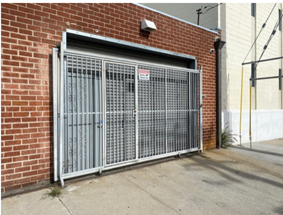
Security exterior equipment entry shipping and receiving point.
