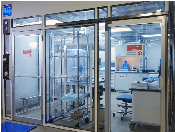
NKC ISO 7 Clean Room
